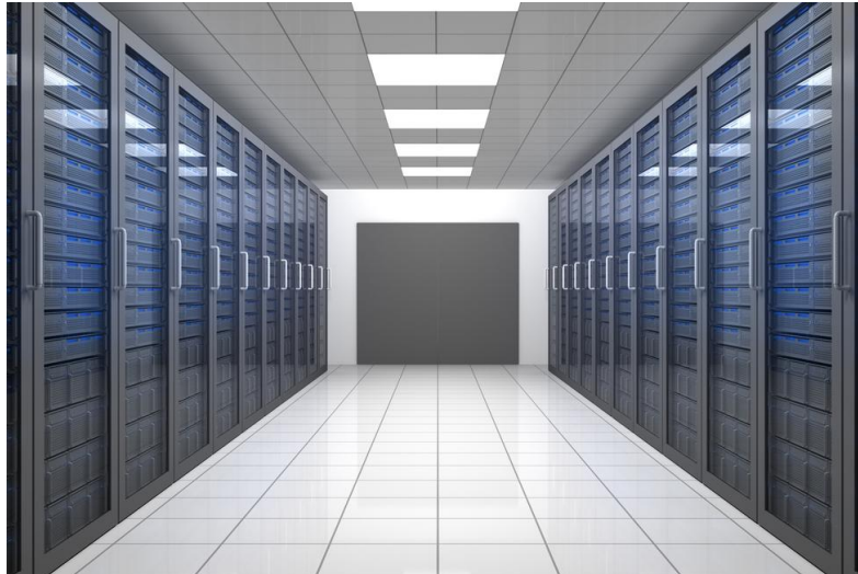
Large datacenter clusters
