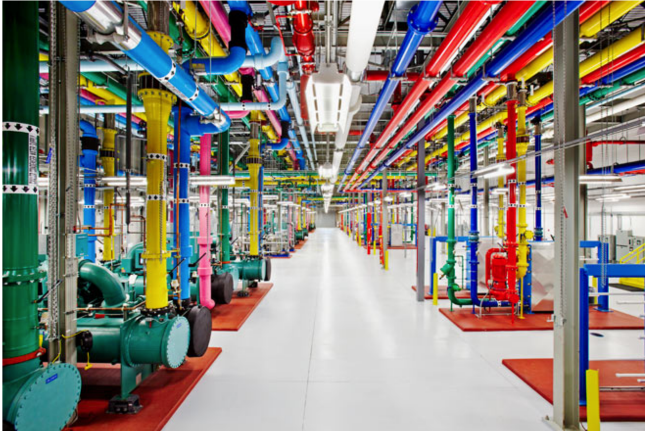
Infrastructure: Cooling systems in Google Datacenter in Georgia
