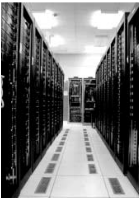
Figure 1: A picture of part of the RCF Linux computing farm at BNL. Two of the networking cabinets can be seen in the background.
